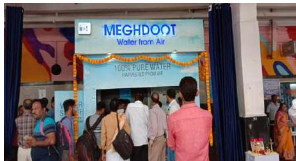
1000 L/day Atmospheric Water Generator Machine installation at Secunderabad Station
