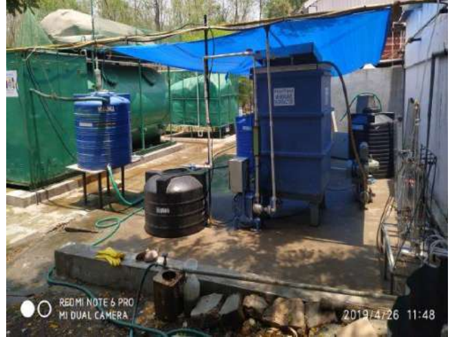
Aerobic Moving Bed Bioreactor (AMBBR) + side stream NF
