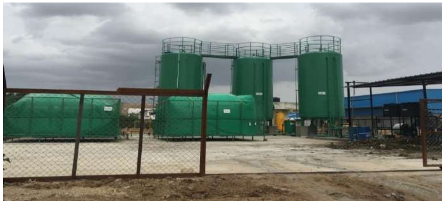
Biogas plant for the treatment of 5000 kg/day of organic fraction of MSW, installed at Jawahar Nagar, MSW Processing Site, Hyderabad
