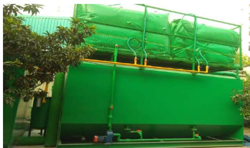
Full scale biogas plant for the treatment of food waste based on AGR at Capgemini, Hyderabad
