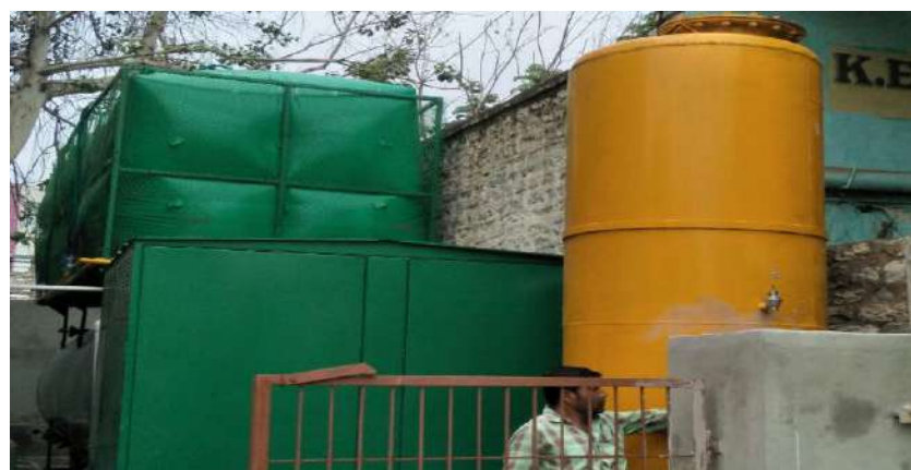
Full scale biogas plant for the treatment of food waste based on AGR at Kurnool, AP
