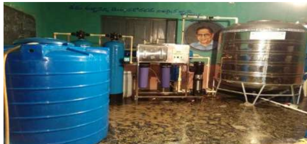
Water Purification Plant (1000 Lit/hr) Installed by IICT at Upper Primary School, Desinenipalem, Khammam District
