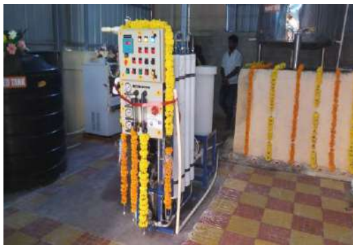
Nanofiltration pilot plant of 1000 L/h capacity installed at Gandhi Hospital, Hyderabad
