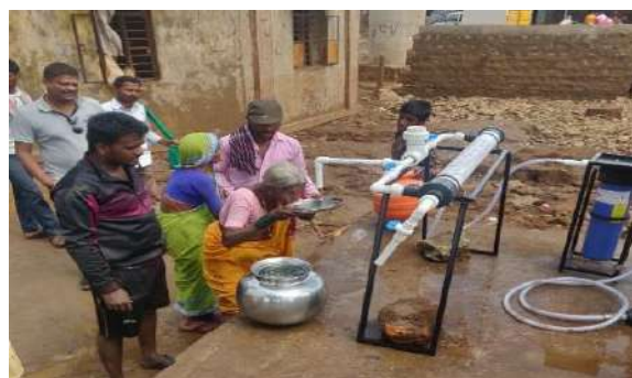
Compact UF plant at Sangli , Maharastra
