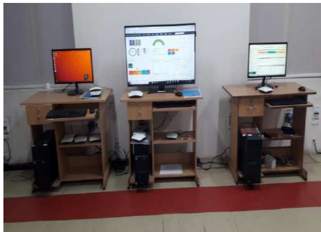
Network Operations Center (NOC)
