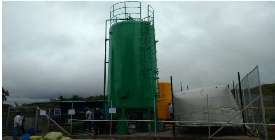
Full scale biogas plant for the treatment of food waste based on AGR at Hubli, Karnataka
